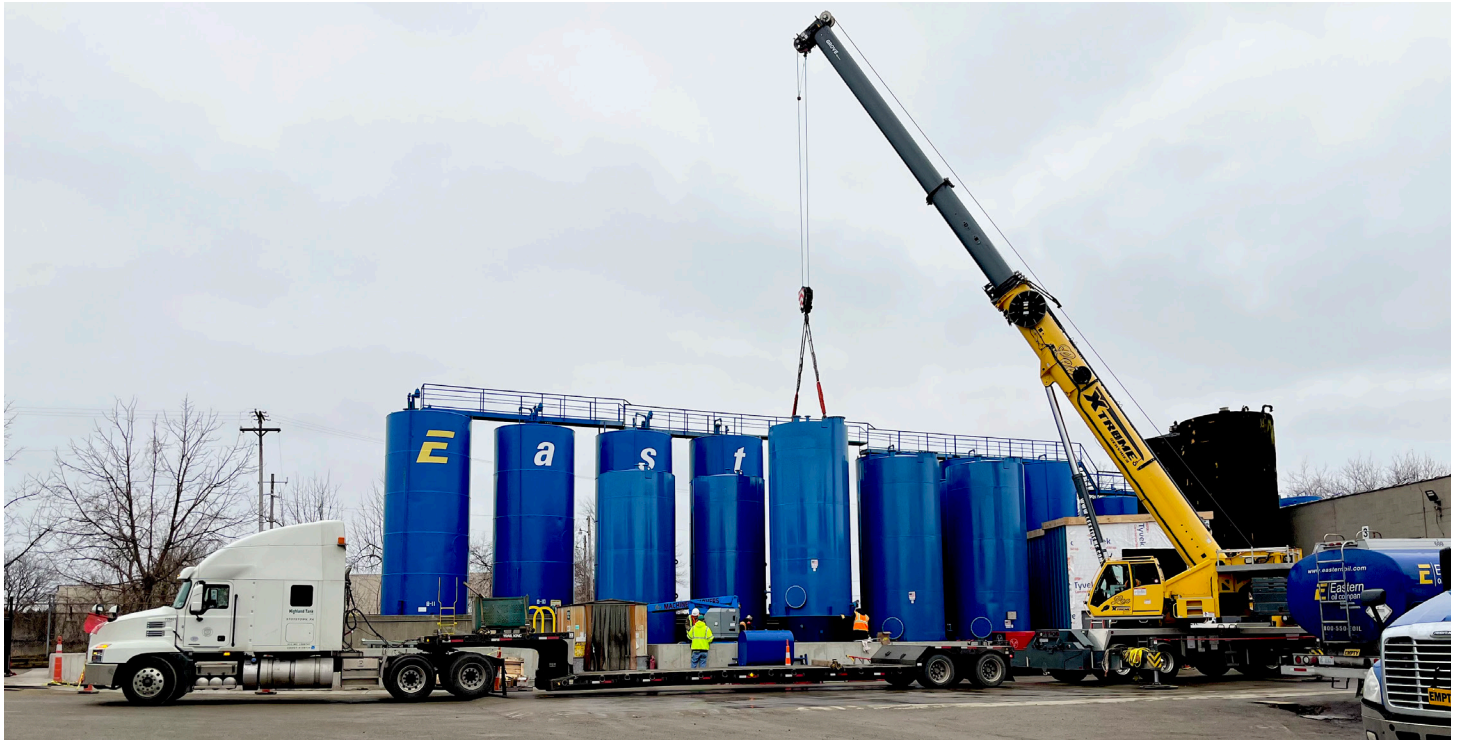
10,000 gallon storage tanks for bulk oil storage and blending
