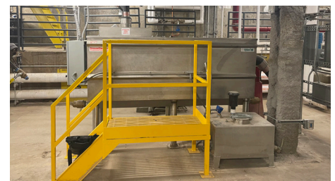
200 GPM Automatic Grease Interceptor at hospital
