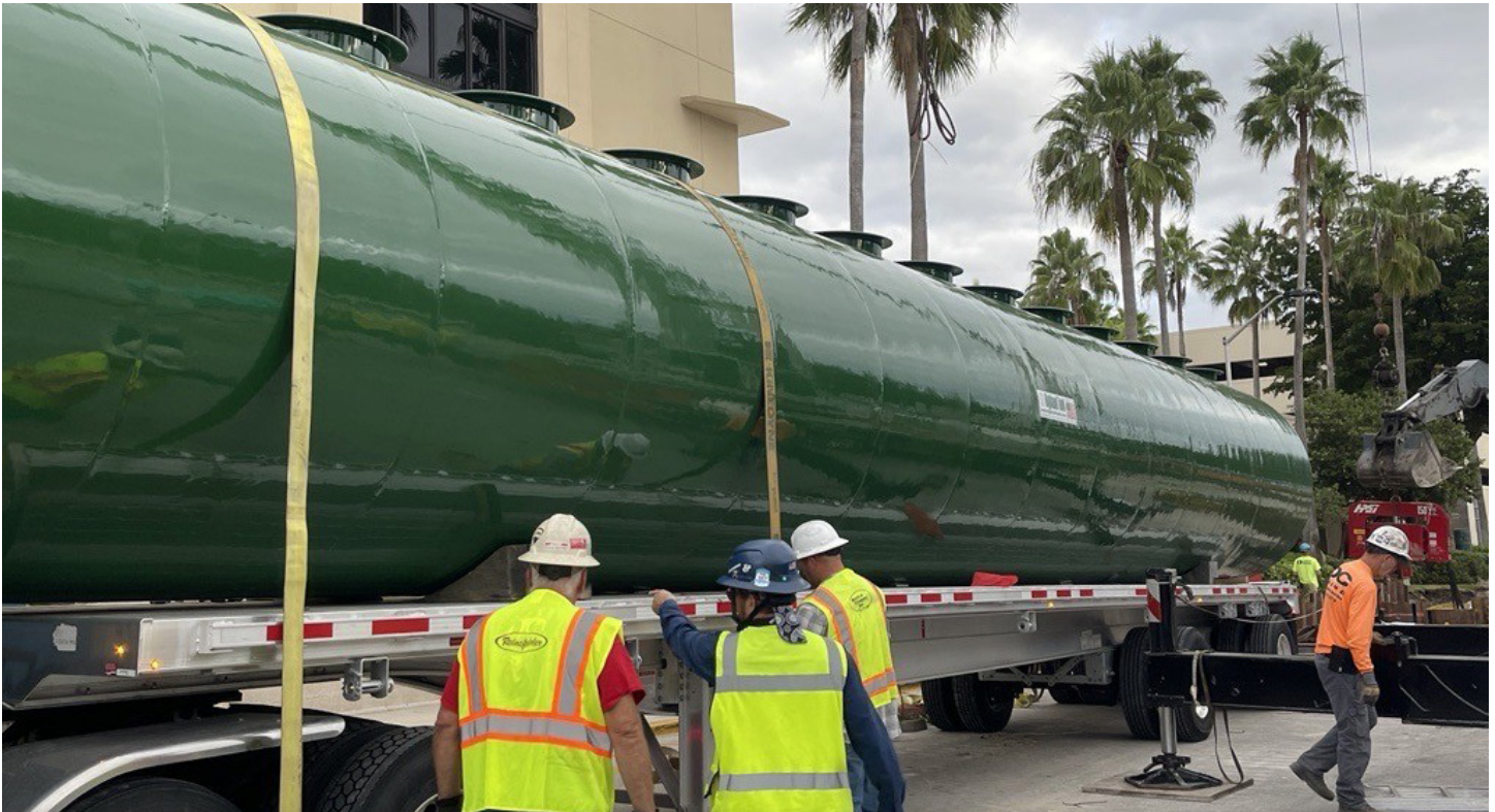
17,500 gallon Passive Grease Interceptor at hospital
