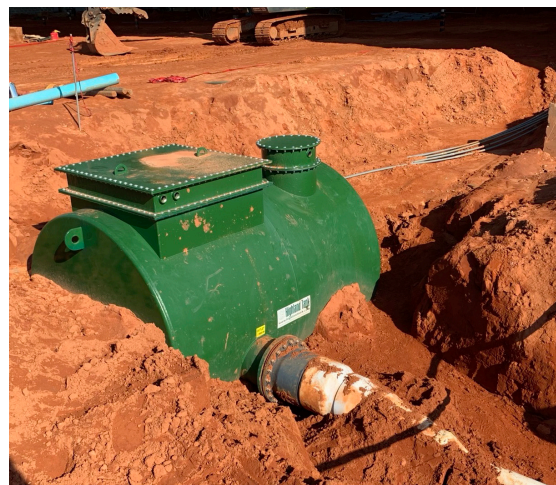
Valve containment tank
